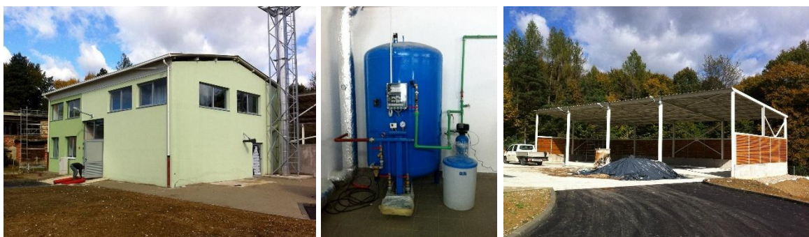
Sl. 6–7 Toplovodna kotlovnica, kotao i spremnik biomase u Pokupskom
